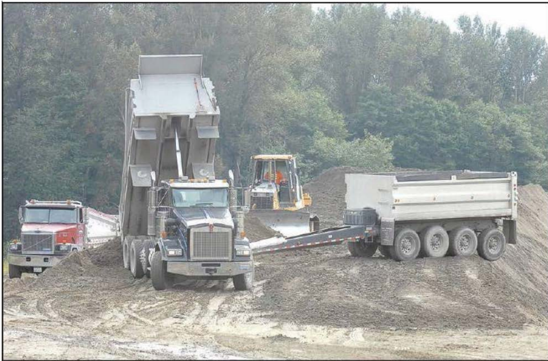
Scott Terrell / Skagit Valley Herald Workers spread part of about 50,000 cubic yards of fill along an existing levee Wednesday along the Skagit River, east of Gardner Road. The Dike District 12 project is being done now so that the fill will be on hand to shape the dikes along the river in the future.
