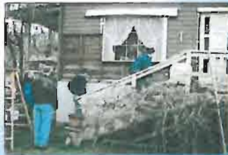
Ripple House #1 with exterior siding removed for inspection of interior wall cavity. First floor elevation 185.51
