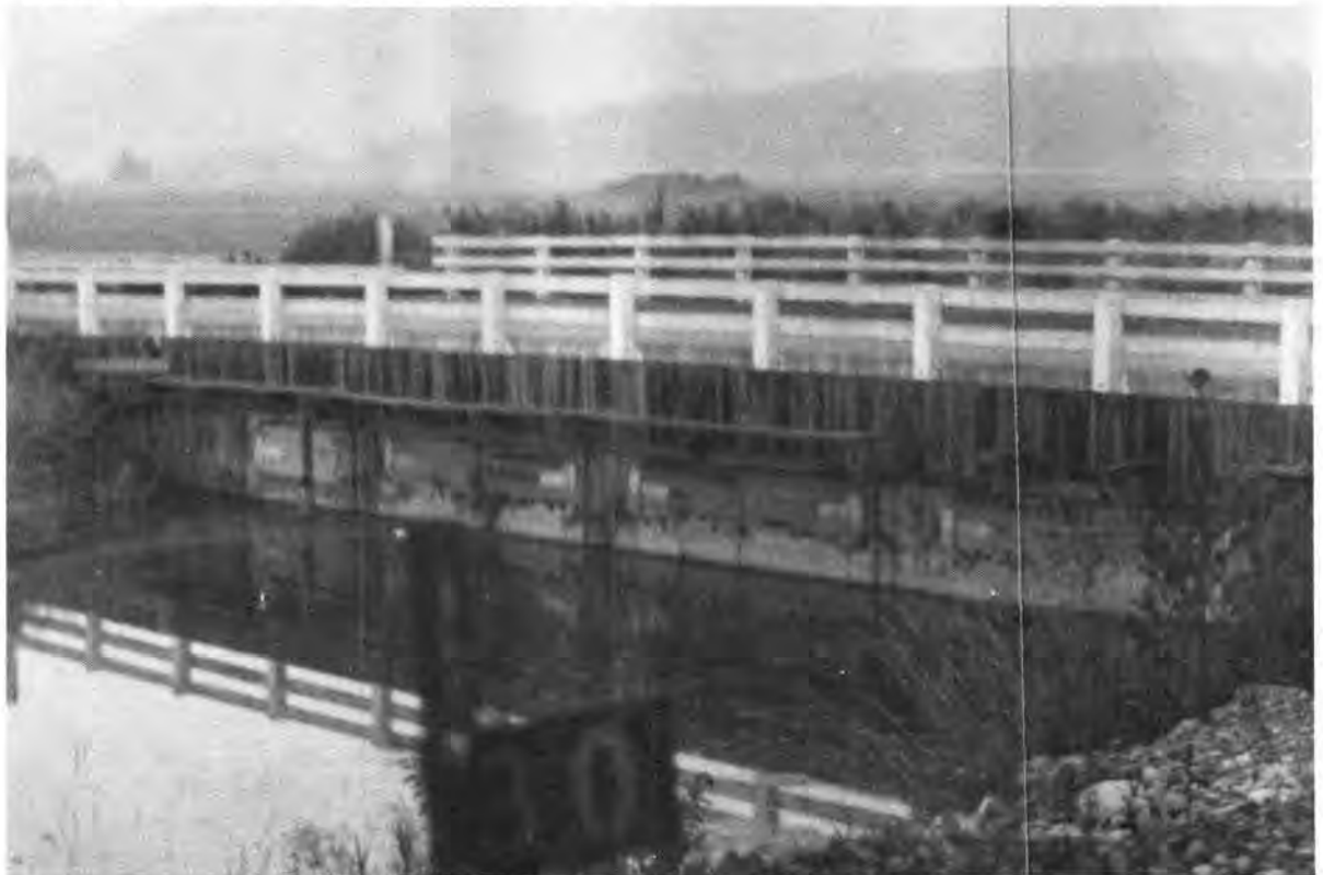
Photo 4-3. View of existing tide gate at Fisher Slough looking east. This structure will be removed and a slide-gate structure constructed closer to the mouth of Fisher Slough.
