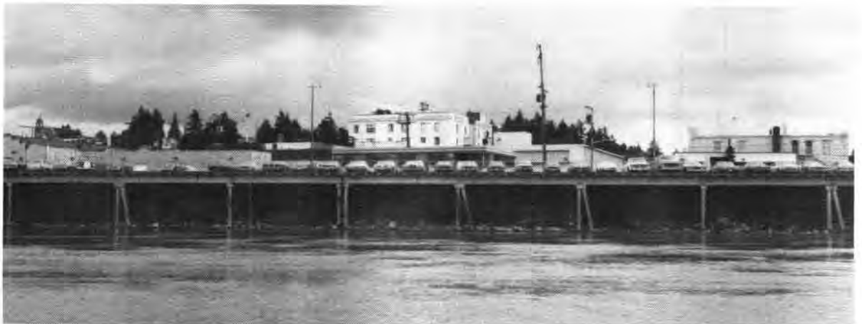
Photo 1-4. View of left bank, Skagit River, through Mount Vernon, looking at the overhanging revetment parking lot. In this particular reach, an aggregate concrete blanket will be utilized under the parking lot rather than rock riprap. A weighted riprap toe will be provided, and a floodwall will be constructed through the parking lot, as illustrated in figure 1-7.
