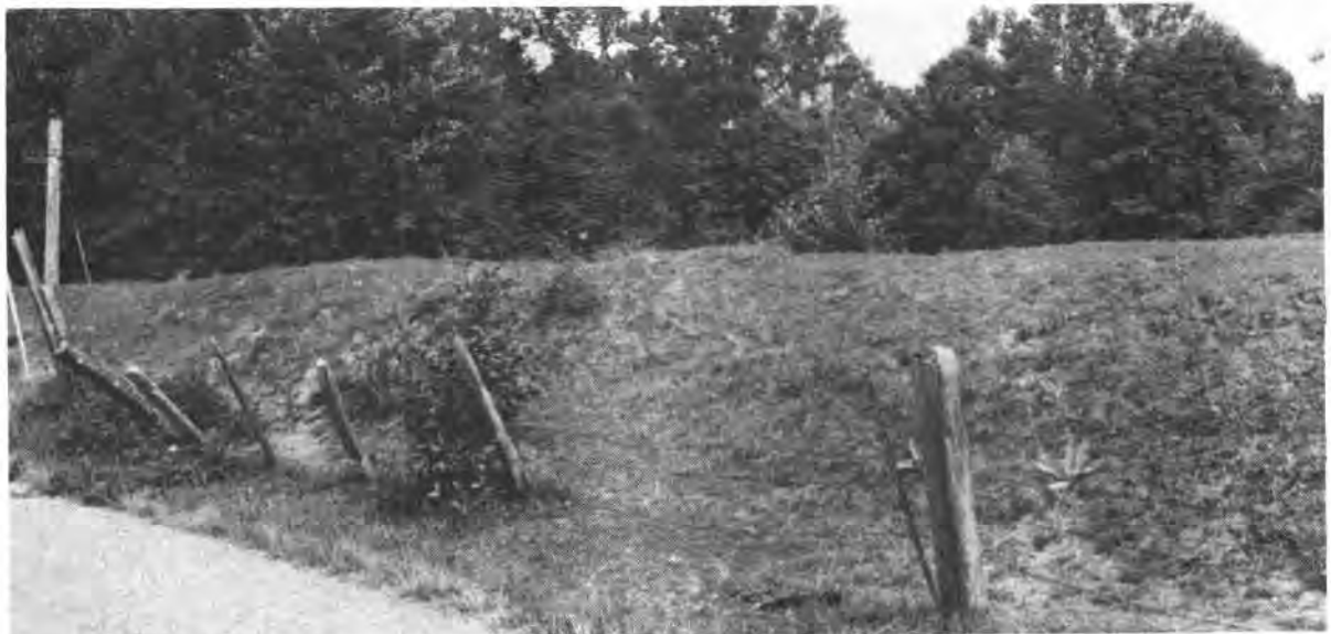
Photo 1-1. View of existing levees on right bank Freshwater Slough, South Fork. Figure 1-3 is typical of levee improvements to be made.
