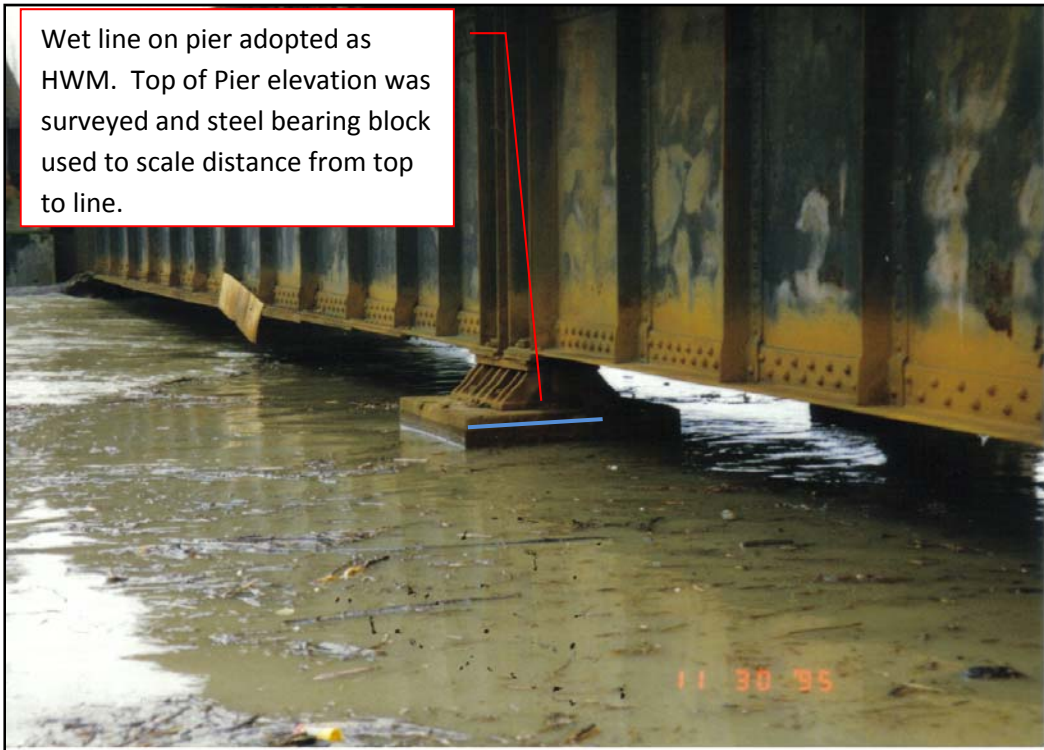
Figure A-4: Close up of BNSF Bridge Pier during November 1995 flood (photo by Chuck Bennett, Dike District 12, courtesy of www.skagitriverhistory.com )
