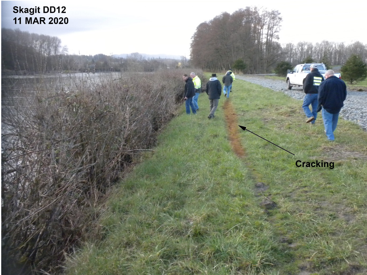
Figure 4. DD 12 cracking along the riverward bench.
