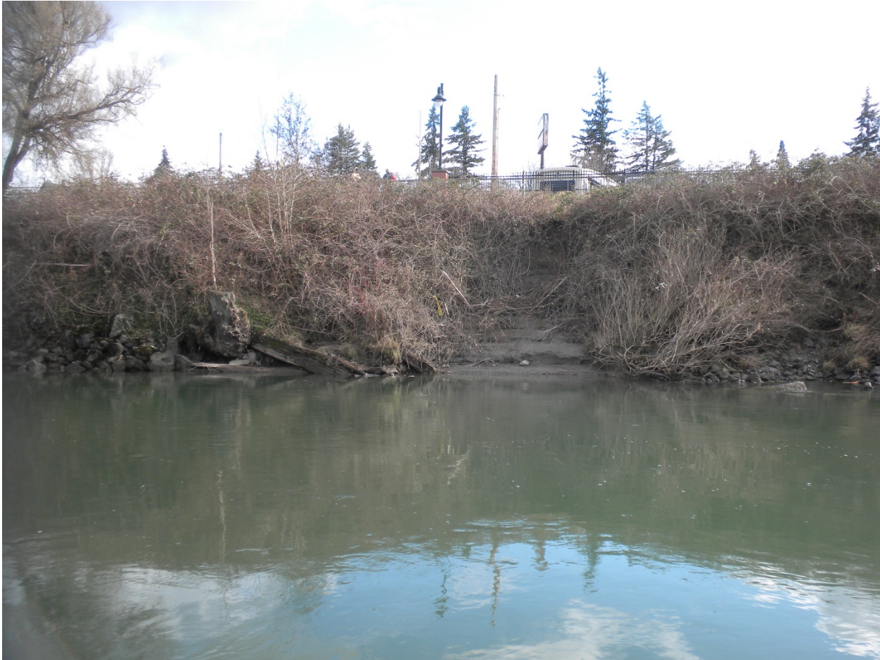
Figure 1. DD 3 repair site showing slope failure.
