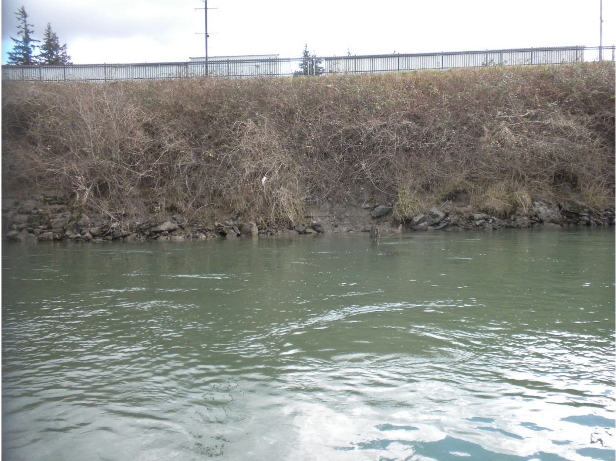
Figure 2. DD 3 damaged segment scour.
