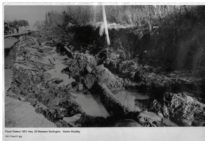
1951 Flood Damage between Burlington & Sedro-Woolley on Highway 20 Picture courtesy Roger Fox Collection
