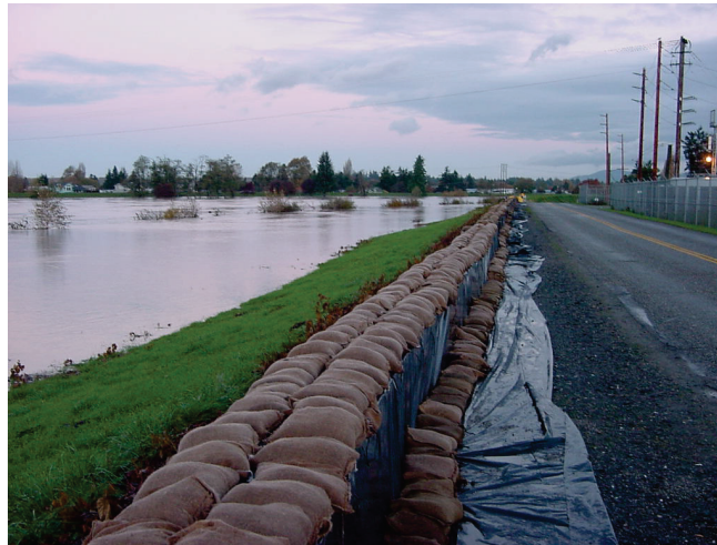
Flood Fighting Efforts to Save Water Treatment Plant Picture courtesy Willy LaRue, City of Anacortes
