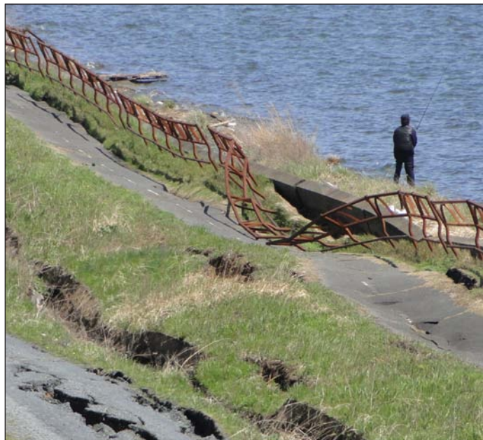
27 April 2011: View of Slumped Hinuma River Left Levee Induced by Liquefaction
