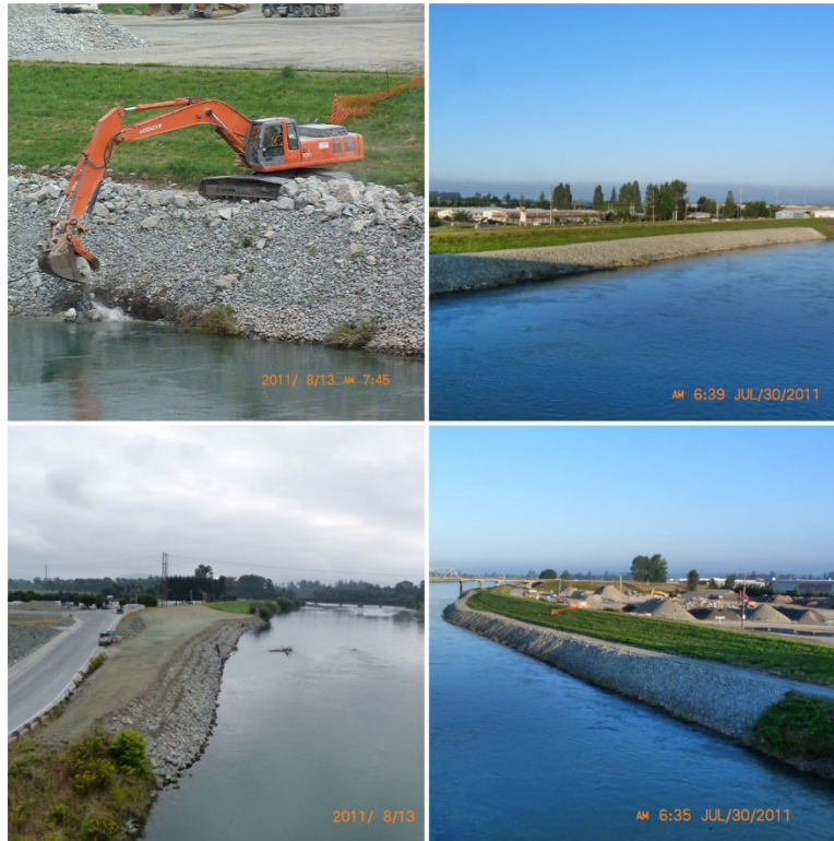
Collage of four 2011 photos taken by SkagitRiverHistory.com of 3 Bridge Corridor Levee Repair Work
