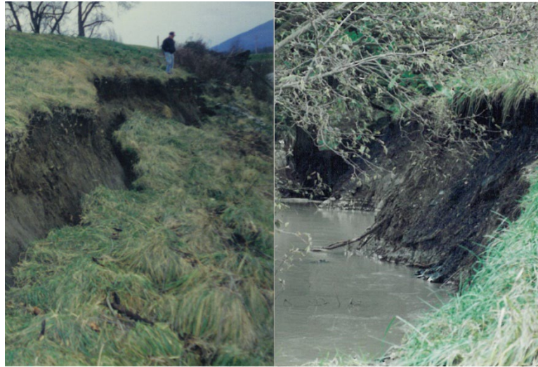
1995 flood damage Dike Dist. 12 levee-bank off Bennett Rd
