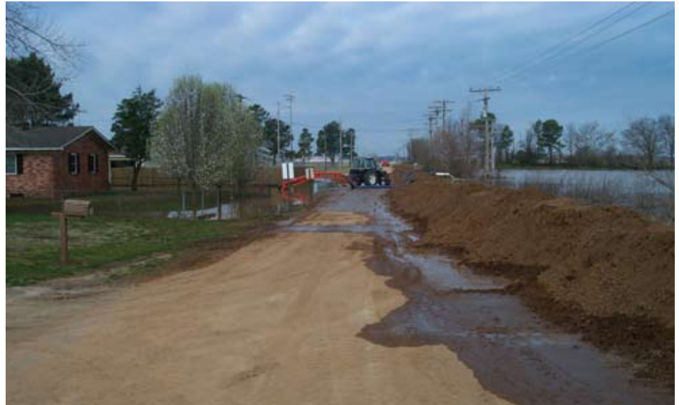
Pumping water out of subdivision after levee breach repaired. Pocahontas, AR. Photo by Elmo Webb, PE 3/23/08
