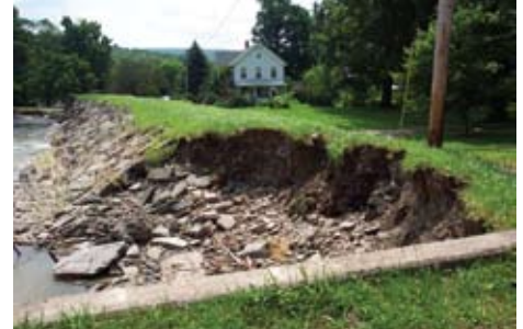
Flood damaged levee, Bainbridge, New York—Courtesy of NYSDEC
