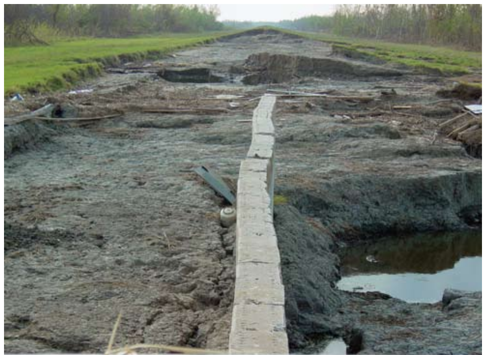
Levee Damaged Due to Overtopping Hurricane Katrina (August 2005) St. Bernard Parish, Louisiana
